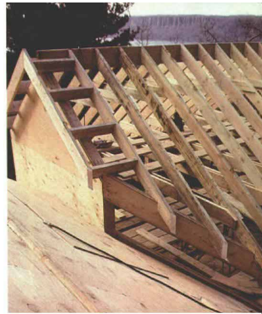
Gable overhang. The gable walls were shortened an extra few inches to allow for 2x10 lookouts, which cantilever beyond the walls to form the overhang. This framing assembly is called a ladder.
